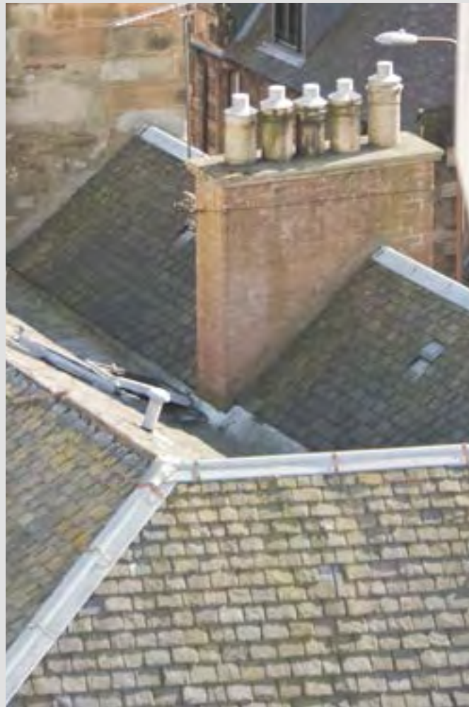
Traditional roofing materials (right) Slate, Lead and zinc are traditional roofing materials used in Edinburgh—seen here from the Museum of Scotland’s roof
