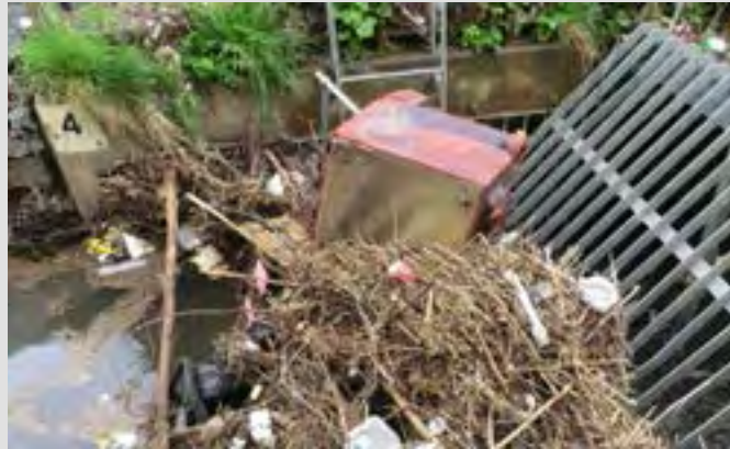
locked up culvert
